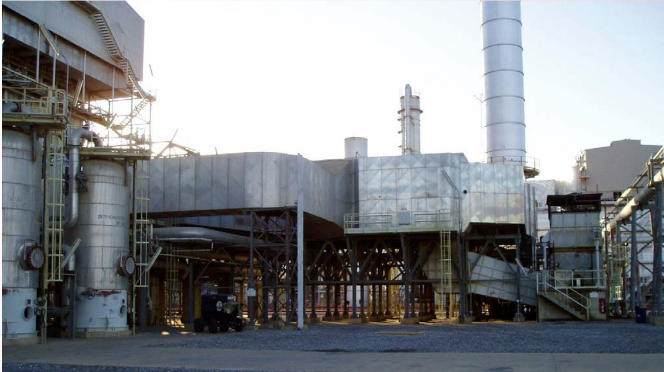
Venezuela, combustion air preheater assembled (SUPERMETHANOL)
