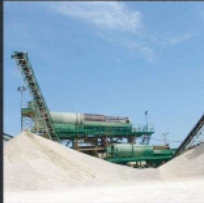
Washing plant of inerts
