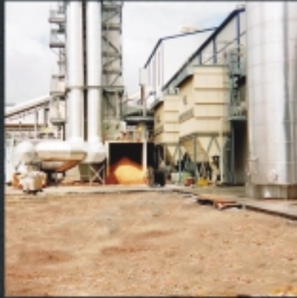
Complete view of the plant
